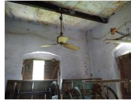
Cracks in ceiling
