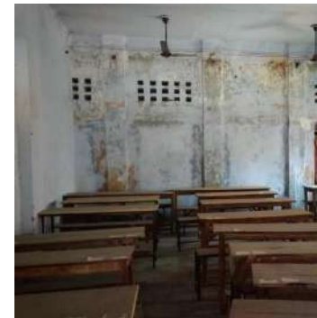
Dampness & water seepage
