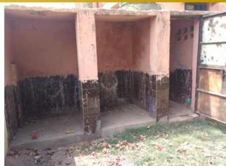
Toilets are in very bad condition need to be repair.
