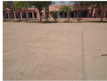
Cracks in basketball court
