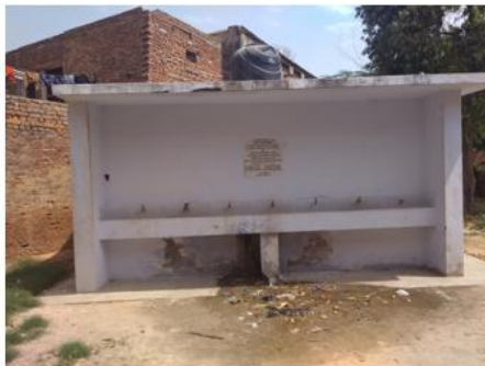
No R.O. is installed for drinking water in the school.
