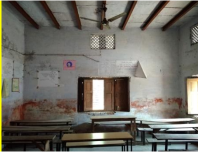
Dampness & Water Seepage
