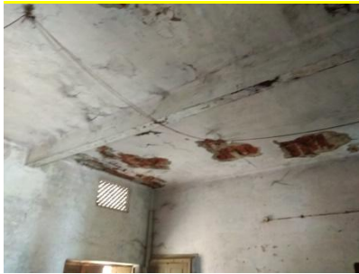
Cracks in ceiling
