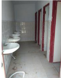
No urinals in boys toilet
