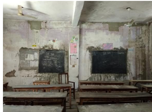
Black Board Damage due to Dampness
