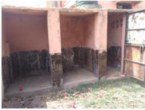
Staff Toilets are in very bad condition
