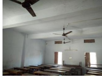
Irregular arrangement of ceiling fans
