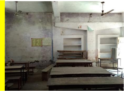
Cracks on wall
