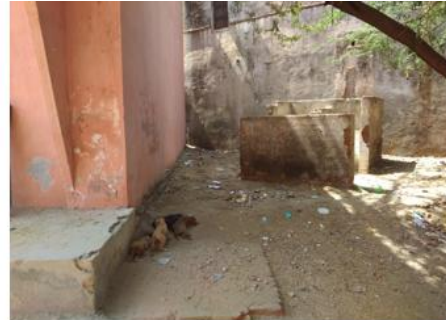
Toilets is in bed condition & not in use today
