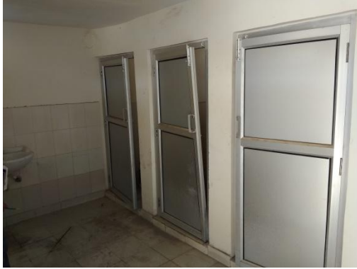
Condition of Toilets doors
