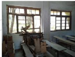
All class windows are damage & no mosquito net
