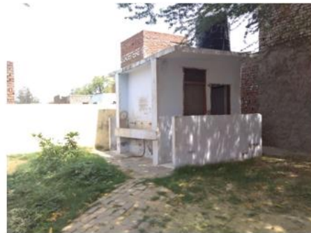
Girls toilet is in bed working condition
