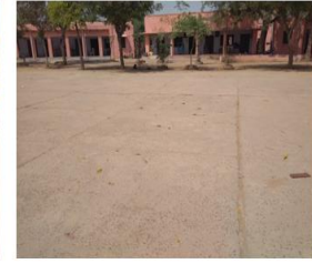
Cracks in basketball court
