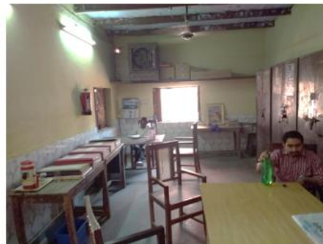
Ceiling and wall of staff room is damage by dampness and need proper maintenance of it
