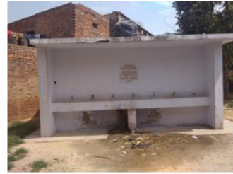
No R.O. is installed for drinking water
