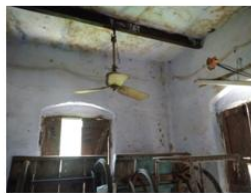
Cracks in ceiling
