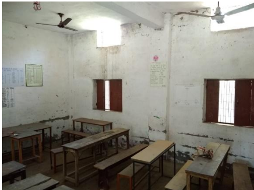
Furniture is in bad condition
