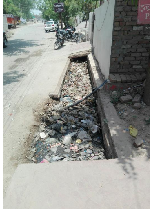
Right side-Chainage 0m to 60m The drain is open and filled with solid waste Needs desilting, raising of side walls and cover slab
