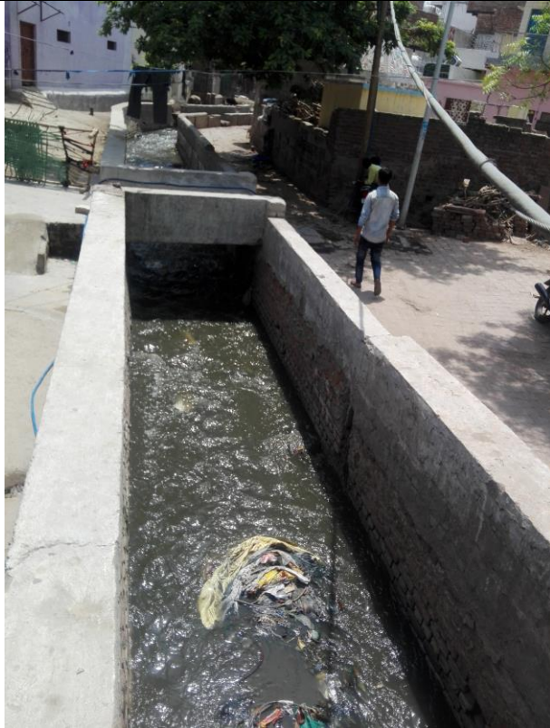
Chainage 2190m to 2340m The drain is open, heavily silted, protection wall needs to be raised and uncovered
