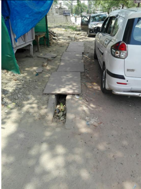
Left side-Chainage 0m to 60m The drain is damaged and filled with soil. Needs desilting, raising of side walls and cover slab
