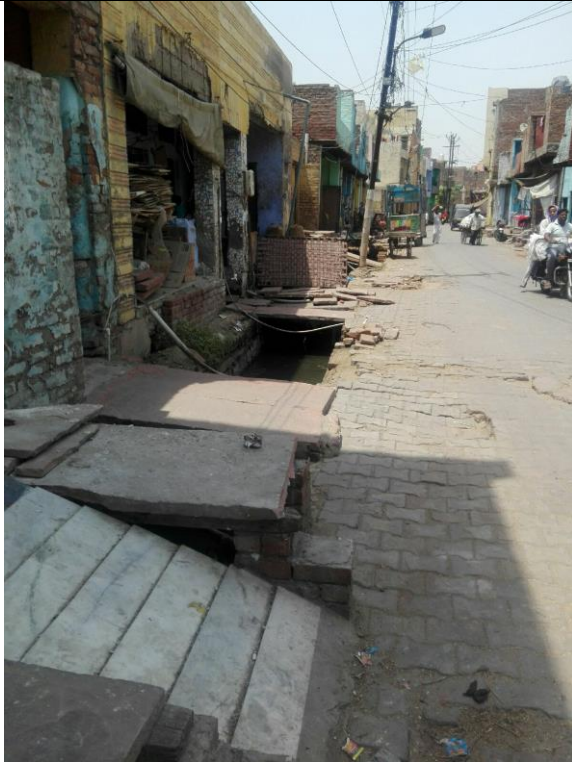
Left side-Chainage 1520m to 2040m Open drain with exposed brick work heavily silted and partially covered by residents
