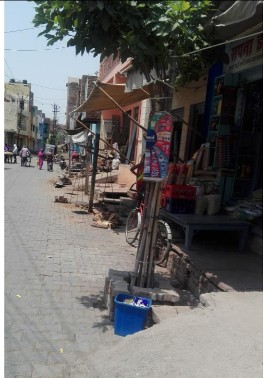
Right side-Chainage 1520m to 2040m The drain is open, heavily silted & exposed brickwork
