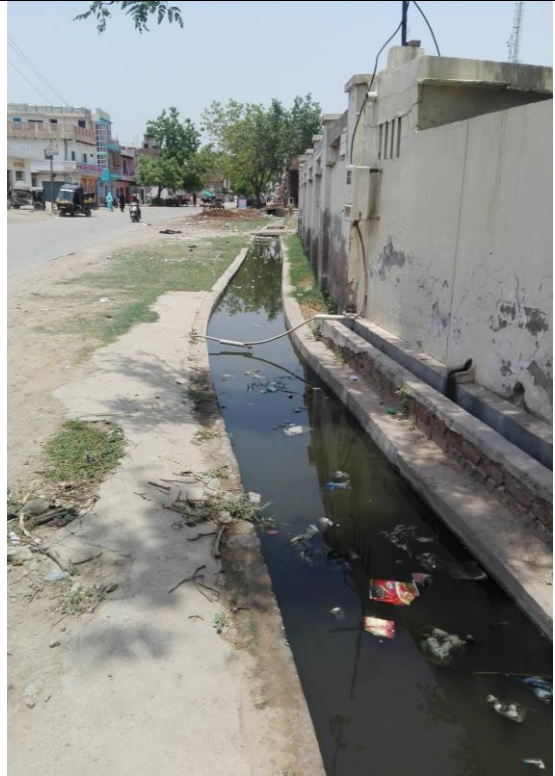
Right side-Chainage 300m to 520m The drain is open, silted
