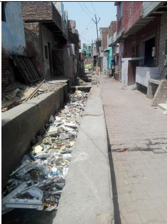
Chainage 2040m to 2130m vulnerable for flooding The drain is open, filled with solid waste, silted exposed brickwork without cover slab
