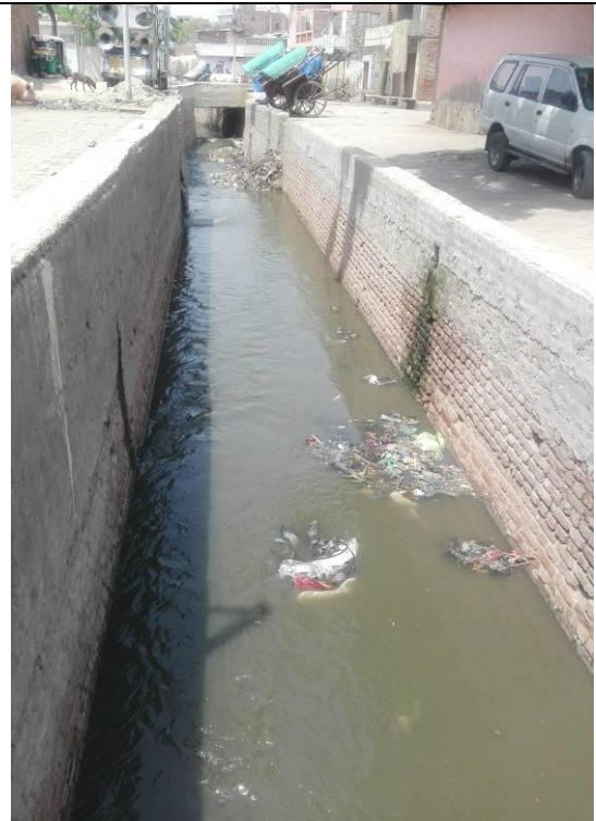
Chainage 2450m to 2820m Open exposed brickwork drain, Desilting, Protection walls need to be raised, cover slab to be provided
