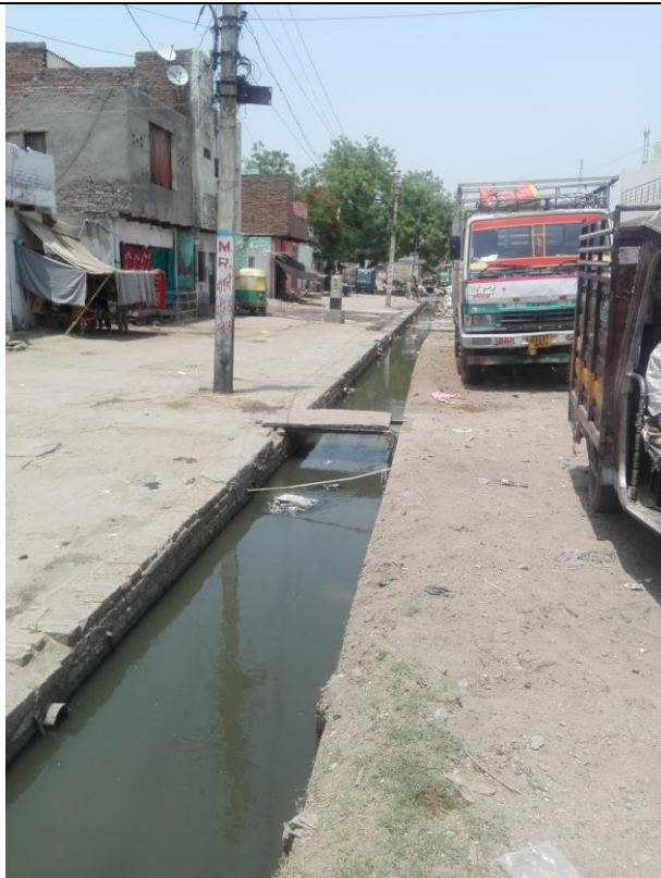
Chainage 810m to 1500m The drain is open, silted & exposed brickwork
