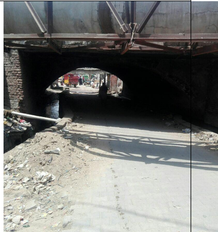
Chainage 1520m Fatebad road junction The drain is open, silted & exposed brickwork
