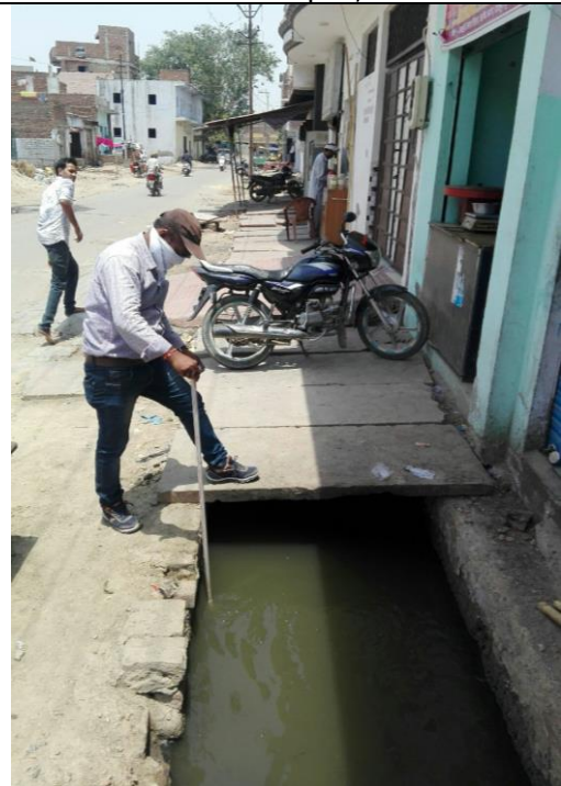
Right side-Chainage 520m to 600m The drain is open, heavily silted & exposed brickwork
