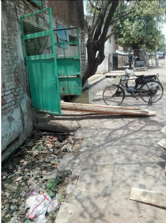
Left side-Chainage 300m to 520m The drain is open, silted and filled with solid waste
