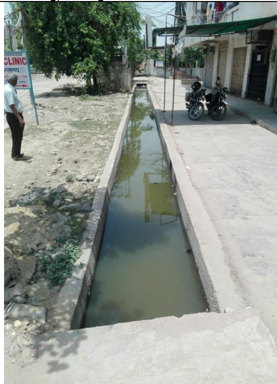
Right side-Chainage 90m to 300m The drain is open, silted. Needs desilting, raising of side walls and cover slab
