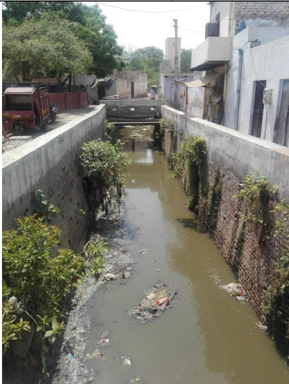
Chainage 3030m to 3090m Open drain with weeds on side walls of drain, Protection wall to be raised and covered with slab
