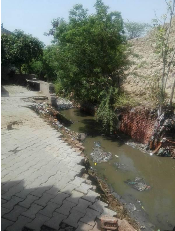
Chainage 2820m to 2910m Open drain without protection wall, soil from righside slides into drain, Protection walls need to be raised, cover slab to be provided
