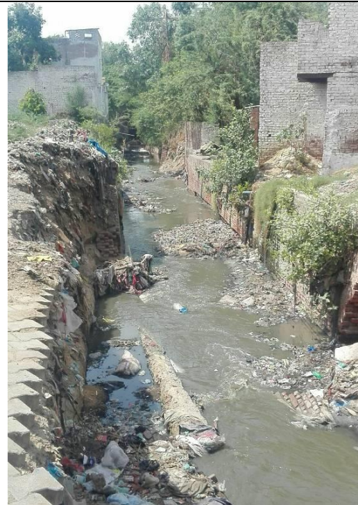
Chainage 3090m to 3180m Open drain in damaged condition, needs desilting, new retining wall in briickwork and cover slab needs to be provided
