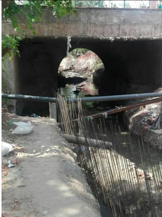
Chainage 3210 crossing near Taj east gate road Open drain without side walls, heavily silted by sliding of soil and needs to be refurbished with brickwork and plasterin
