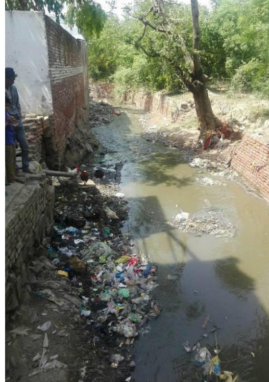
Chainage 2910m to 3030m Open drain side retaining walls are damaged, silted and new retaining walls to be provided with cover slab
