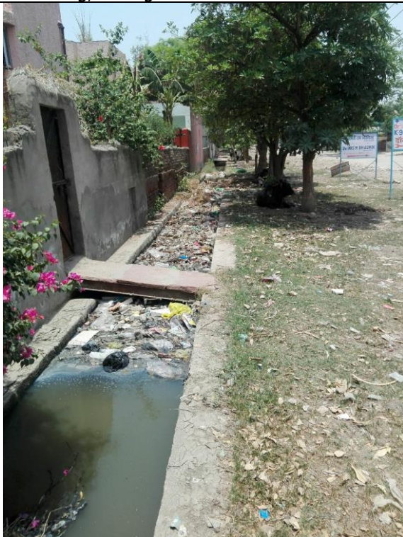
Left side-Chainage 60m to 300m The drain is open, silted and filled with solid waste. Needs desilting, raising of side walls and cover slab
