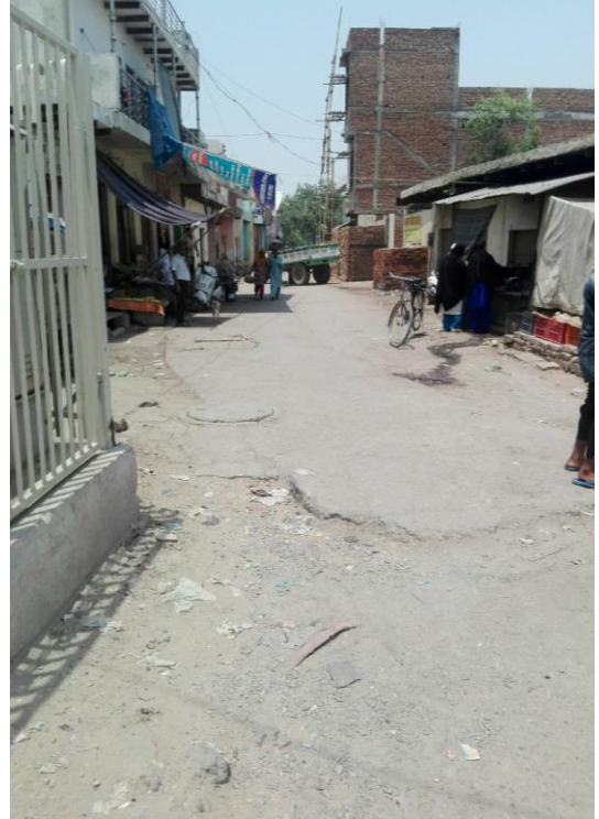
Chainage 680m to 810m The drain is closed with RCC slab and serving as road
