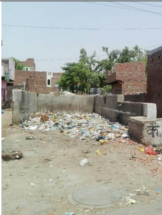
Chainage 2420m to 2450m Road culvert crossing Solid waste dumping yard drain is open, heavily silted, protection wall needs to be raised and uncovered
