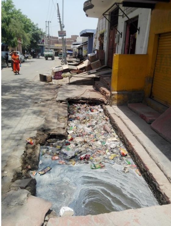
Right side-Chainage 600m to 680m The drain is open, filled with solid waste, heavily silted & exposed brickwork
