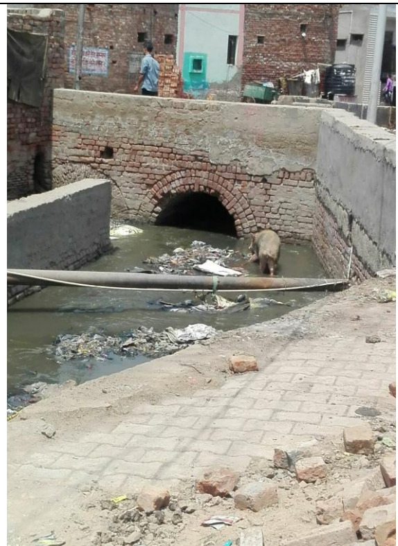
Chainage 2160m to 2190m road crossing The drain is open, heavily silted, no protection wall on sides and no cover slab
