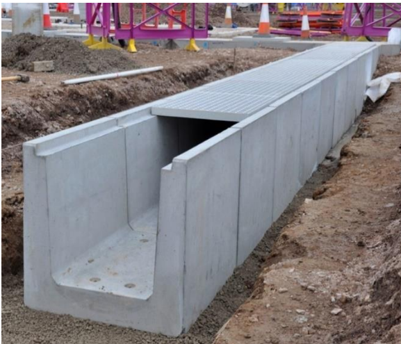
Utility Ducts: For Storm Water & Electrical Cables
