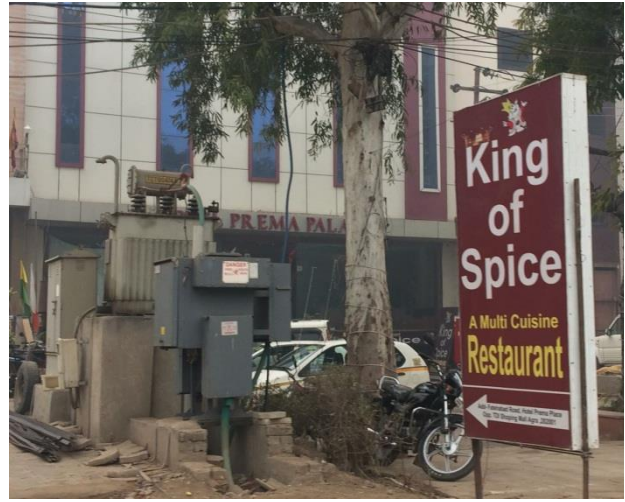
electrical utilities on road
