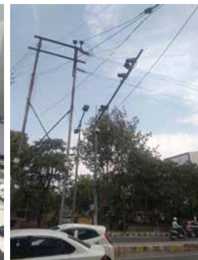
Figure 6. Cameras installed in the junctions, Source: Author
